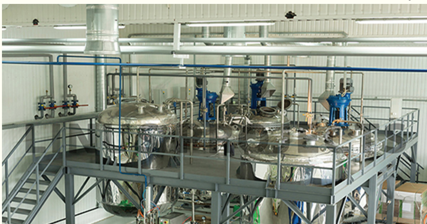
Linus Project - Brake Fluid and Coolant Plant
