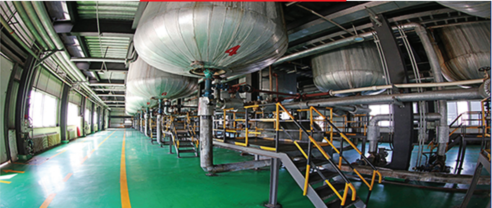
Lube Oil Blending plant
